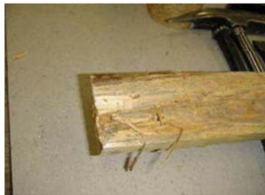
Rotten Wood: Not OK
