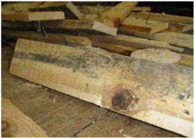
Mold: Not OK
