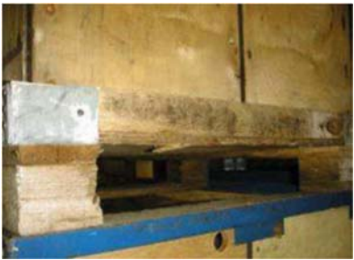
Dampness and Mold: Not OK
