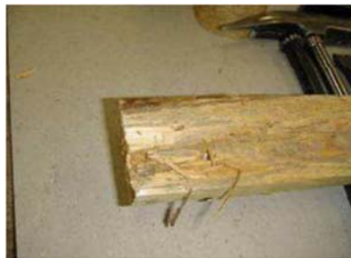
Rotten Wood: Not OK
