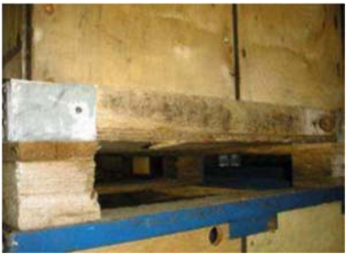
Dampness and Mold: Not OK
