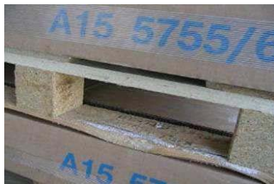
Mold: Not OK
