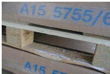
Mold: Not OK
