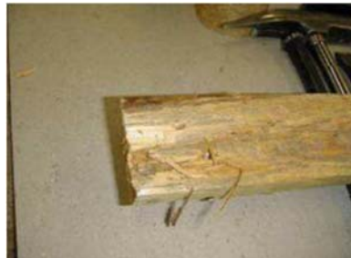
Rotten Wood: Not OK
