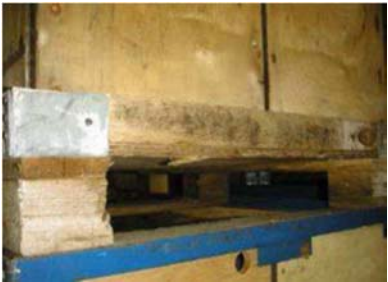
Dampness and Mold: Not OK
