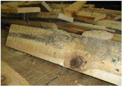
Mold: Not OK
