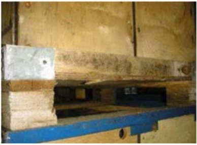
Dampness and Mold: Not OK
