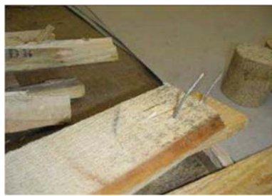
Mold: Not OK
