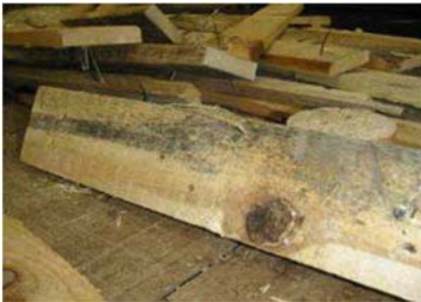
Mold: Not OK
