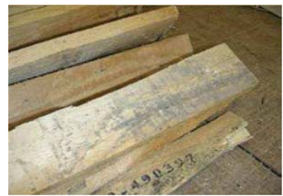
Mold: Not OK
