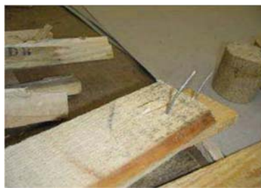
Mold: Not OK
