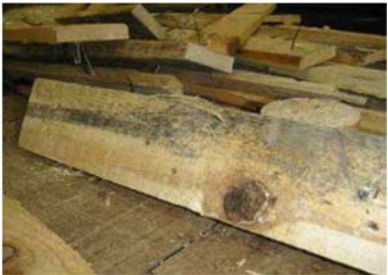
Mold: Not OK
