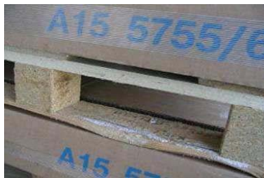
Mold: Not OK
