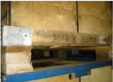
Dampness and Mold: Not OK
