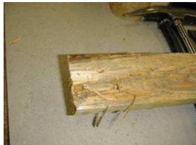
Rotten Wood: Not OK
