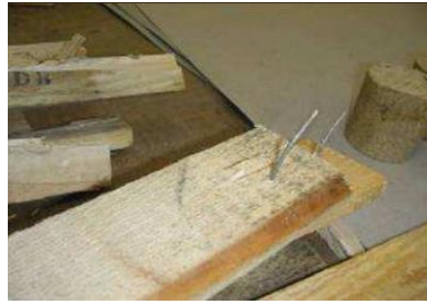
Mold: Not OK
