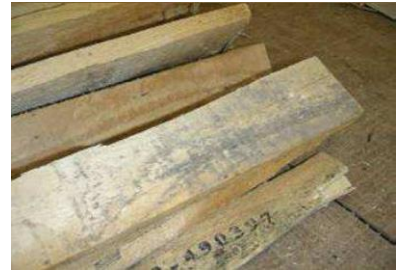
Mold: Not OK
