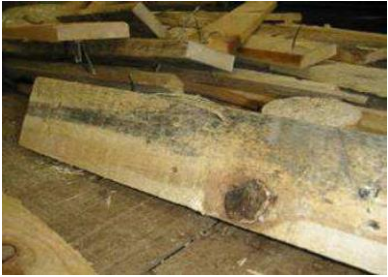
Mold: Not OK
